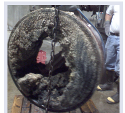
Struvite buildup in a WRF pipe
