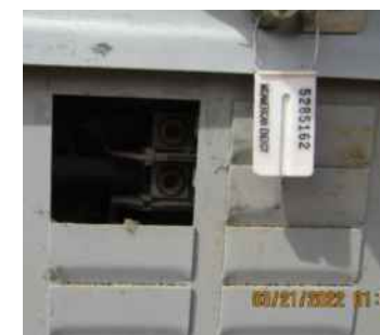
BROKEN MAIN DISCONNECT
